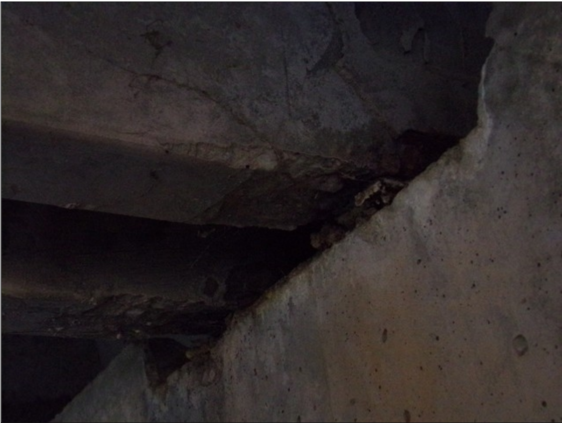
TYPICAL MINOR SPALLING (UP TO 4 INCHES X 3 INCHES X 1/2 INCHES DEEP) WITH NO EXPOSED REBAR TO BOTTOM OF LEGS ADJACENT TO BEARING, SPAN 1 BEAM 3
