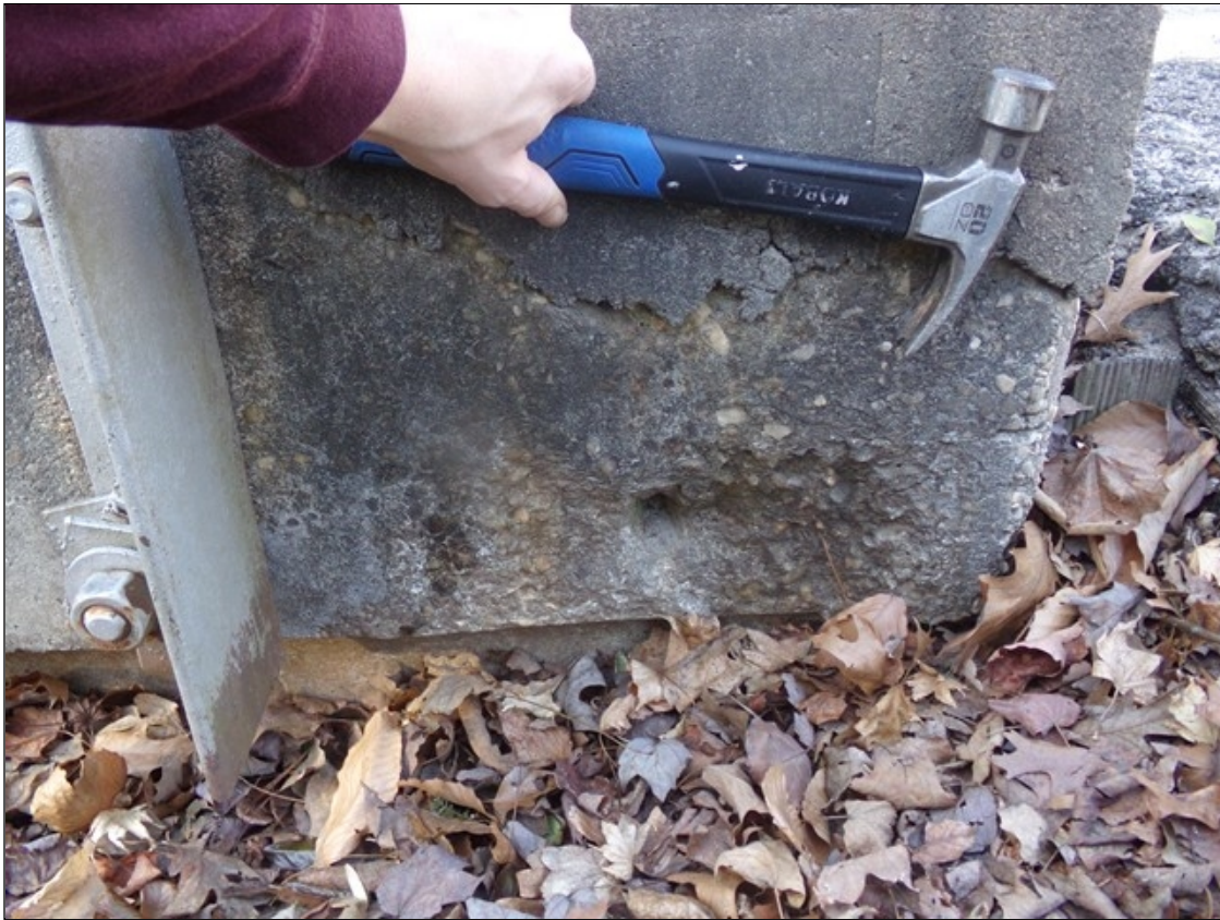
SPAN 3 RIGHT RAIL - SPALL (12 INCHES LONG X 6 INCHES HIGH X 1 INCH DEEP) WITH NO EXPOSED REBAR TO OUTSIDE FACE AT FAR END
