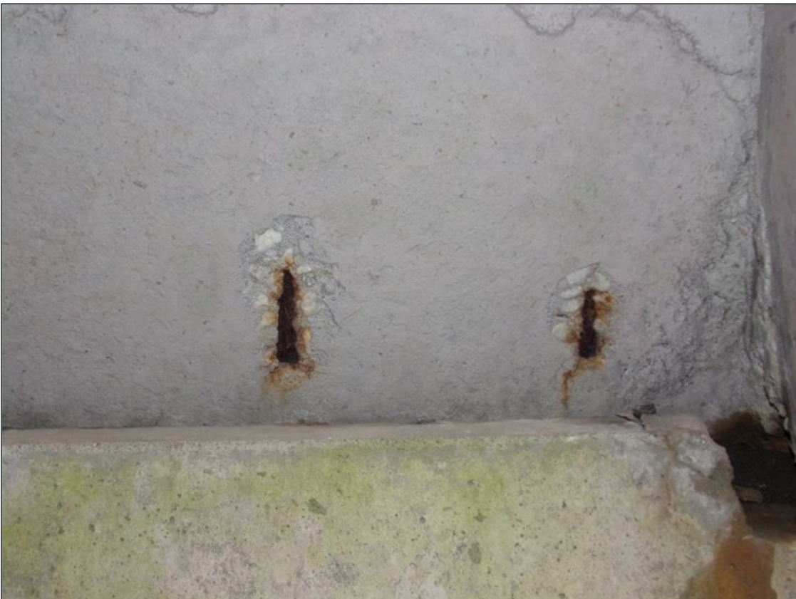
TYPICAL SPALLING (UP TO 8 INCHES X 2.5 INCHES X 1/4 INCH DEEP) WITH EXPOSED REBAR (NO SECTION LOSS) AT DIAPHRAGMS, SPAN 1 BEAM 1 NEAR DIAPHRAGM
