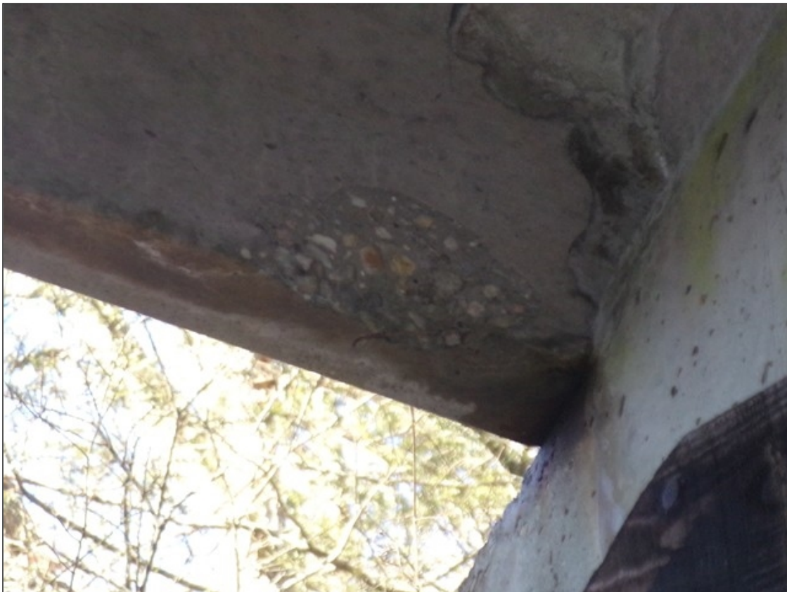
SPAN 2 BEAM 1 - SPALL (8 INCHES X 6 INCHES X 1/2 INCH DEEP) WITH NO EXPOSED REBAR TO RIGHT FACE OF LEFT LEG AT FAR END
