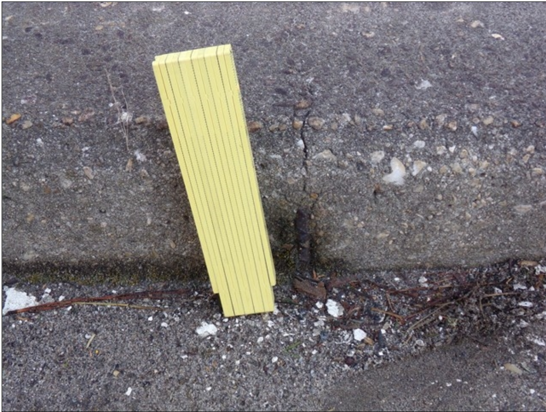
SPAN 3 RIGHT RAIL - EXPOSED REBAR (3 INCHES LONG) WITH NO SECTION LOSS TO INSIDE FACE OF CONCRETE CURB AT MIDSPAN
