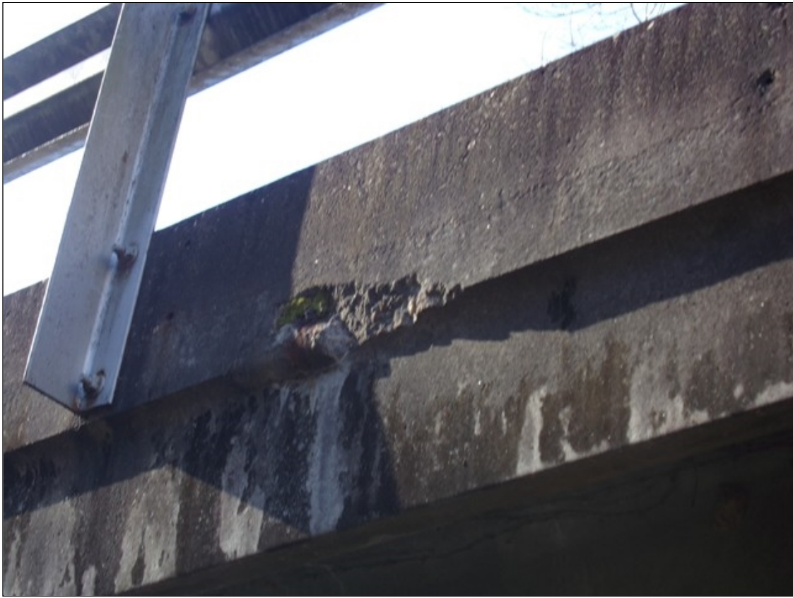
SPAN 2 BEAM 10 - SPALL (12 INCHES X 6 INCHES X 1 INCH DEEP) WITH NO EXPOSED REBAR TO RIGHT SIDE OF TOP FLANGE AT 4 FEET FROM FAR END
