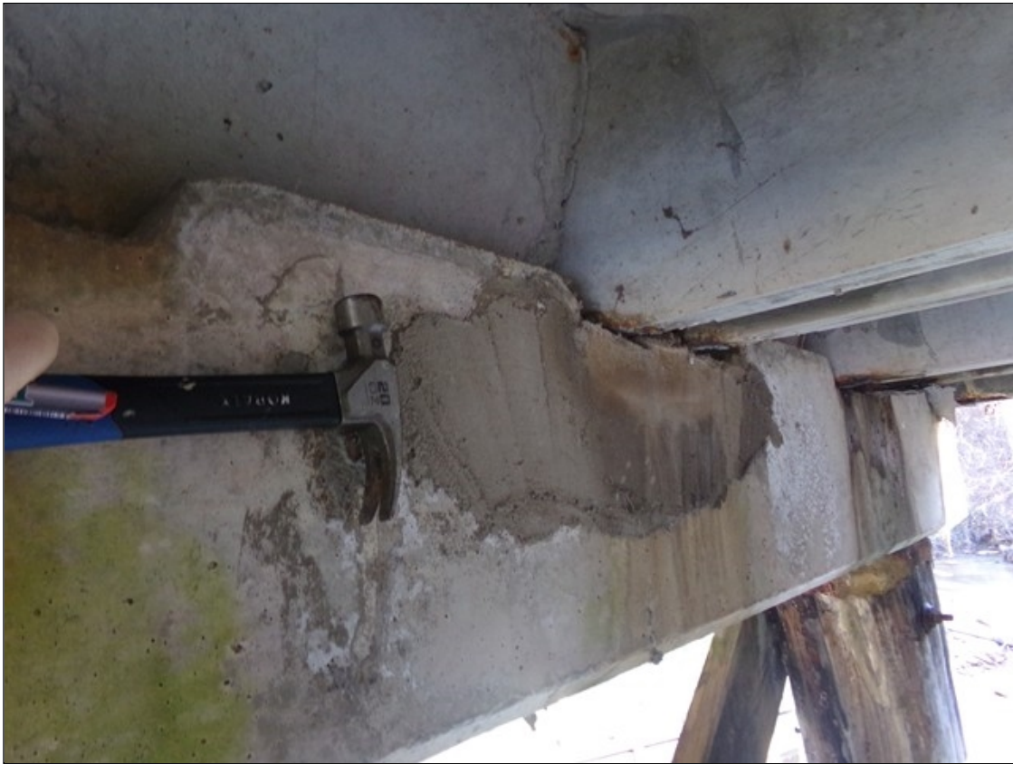
TYPICAL INTERMITTENT SOUND PATCHING (UP TO 24 INCHES X 6 INCHES) THROUGHOUT CAP, BENT 1 NEAR FACE
