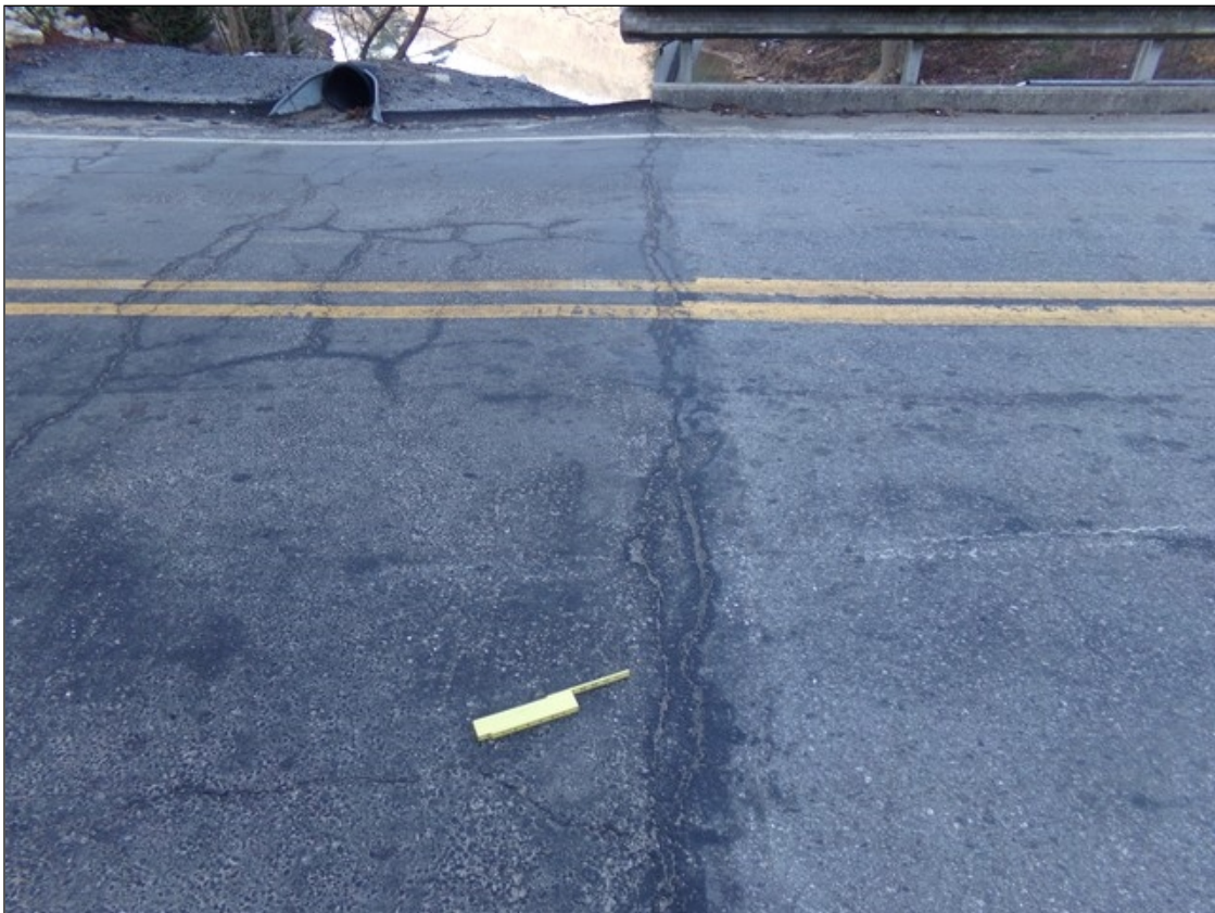
TYPICAL TRANSVERSE OPEN CRACKING (1/2 INCH X FULL WIDTH) TO ASPHALT WEARING SURFACE OVER END BENTS, OVER END BENT 1
