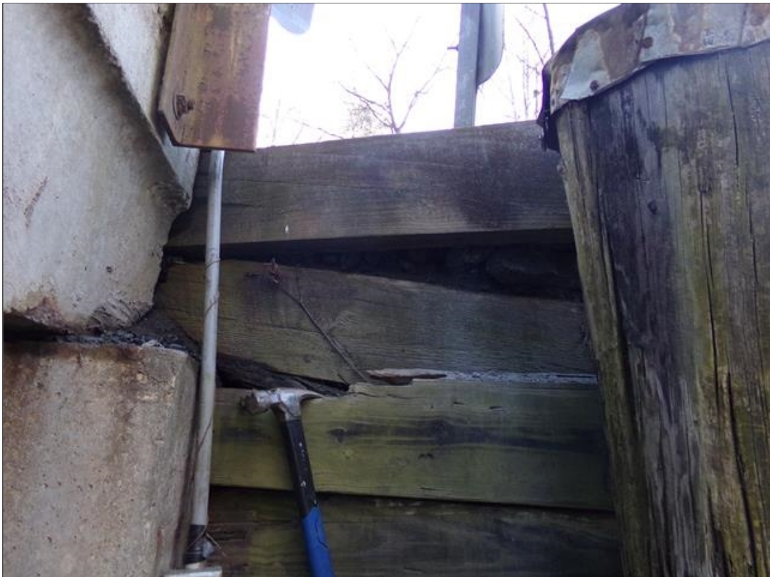
END BENT 1 ABUTMENT - X3 BOARDS LOOSE, NOT CONNECTED TO SOLDIER PILE AND ALLOWING SPILL-THROUGH AT TOP OF LEFT SIDE ABUTMENT EXTENSION (PAR)
