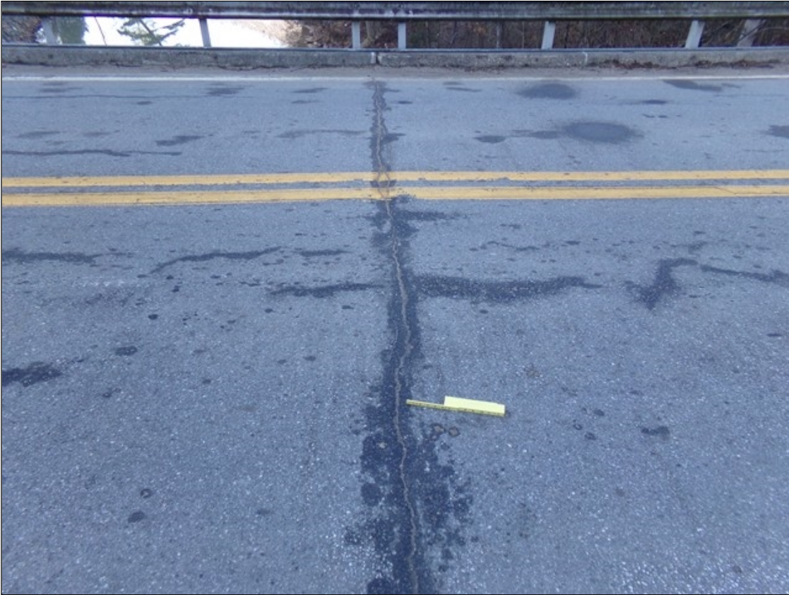
TYPICAL OPEN CRACKING (1/2 INCH X FULL WIDTH) TO ASPHALT WEARING SURFACE OVER INTERIOR BENTS, OVER BENT 1
