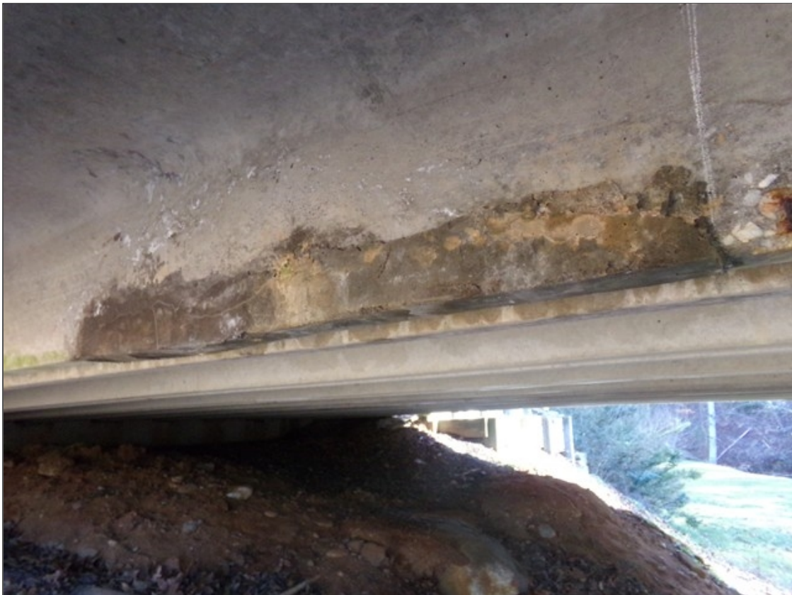
SPAN 3 BEAM 1 - UNSOUND PATCH (30 INCHES LONG X 3 INCHES WIDE X 4 INCHES HIGH) WITH HAIRLINE CRACKING TO RIGHT LEG AT 8 FEET FROM NEAR END
