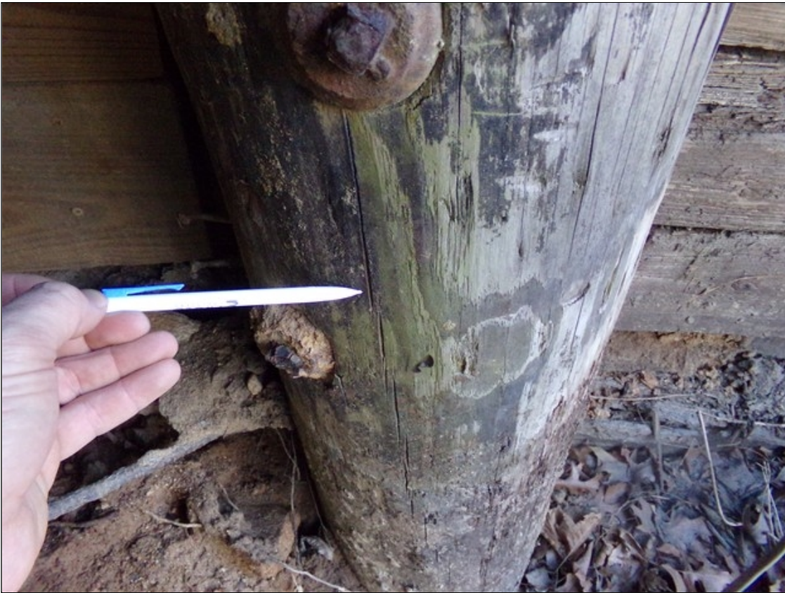
TYPICAL CHECKING (UP TO 1/4 INCH DEEP) THROUGHOUT PILES, END BENT 1 PILE 1
