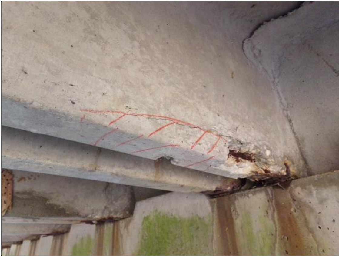
SPAN 3 BEAM 2 - SPALLING / DELAMINATION (18 INCHES LONG X 4 INCHES WIDE X UP TO 2 INCHES DEEP) WITH EXPOSED PRESTRESSING (15 PERCENT SECTION LOSS) TO BOTTOM OF RIGHT LEG AT NEAR END (PAR)
