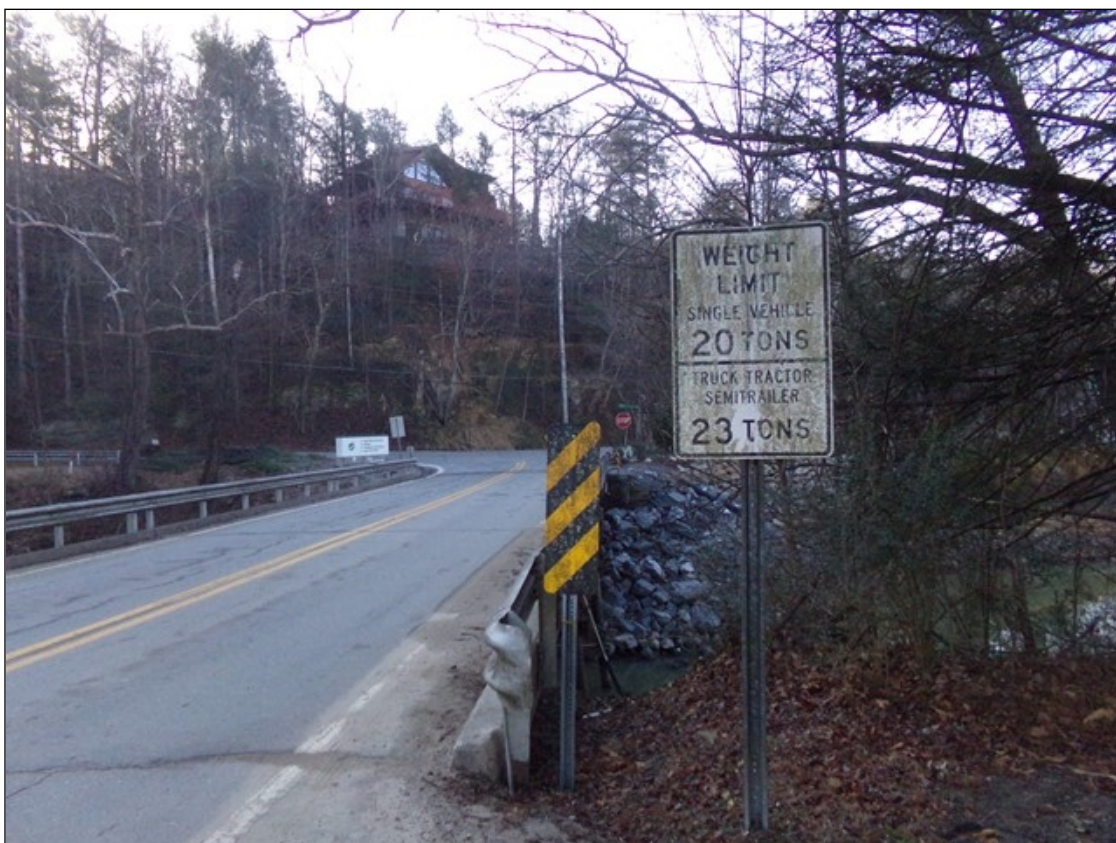
WEIGHT LIMIT POSTING AT NORTH APPROACH
