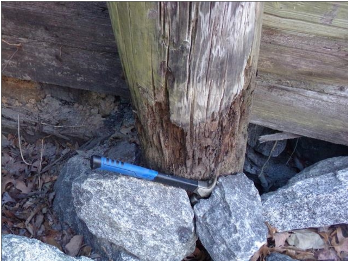
END BENT 1 ABUTMENT - LEFT SIDE EXTENSION SOLDIER PILE - DECAY (UP TO 2 FEET HIGH X 1 INCH DEEP) AT GROUNDLINE AND HOLLOW WHEN SOUNDED (PAR)
