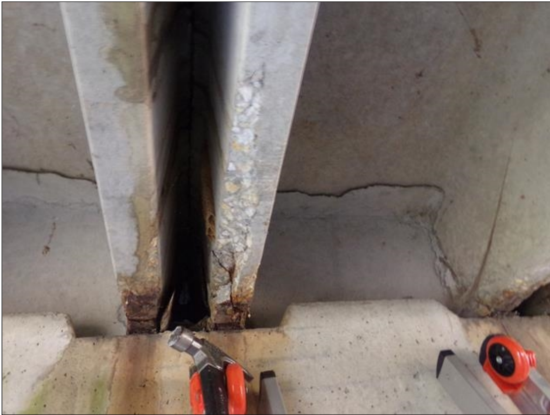
SPAN 3 BEAM 6 - SPALL (20 INCHES LONG X UP TO 3 INCHES WIDE X 2 INCHES DEEP) WITH EXPOSED PRESTRESSING (NO SECTION LOSS) TO RIGHT LEG AT NEAR END (PAR)
