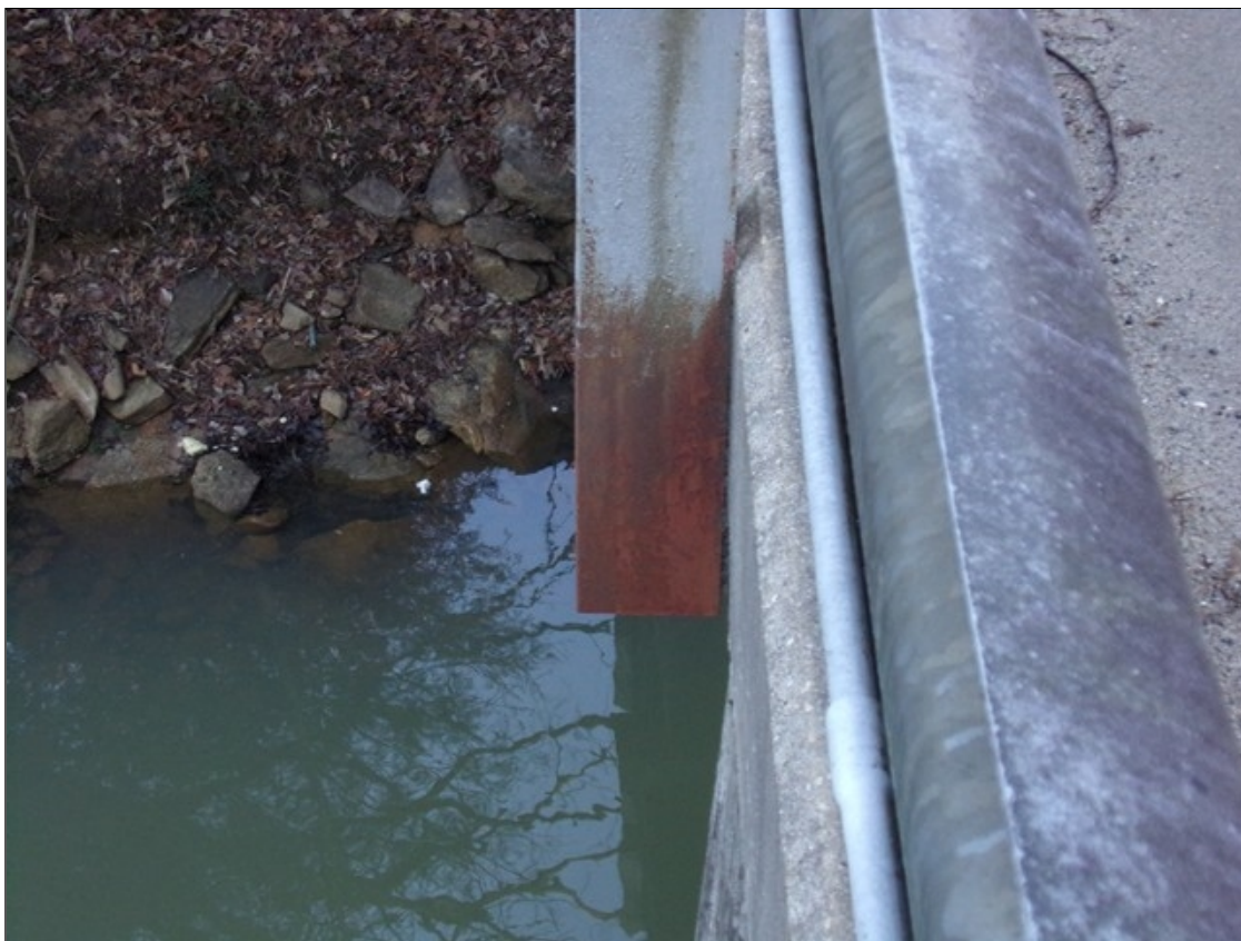
TYPICAL MODERATE SURFACE CORROSION AT RAIL POSTS, SPAN 1 POST 5
