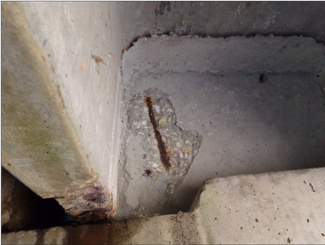
TYPICAL SPALLING (UP TO 8 INCHES X 4 INCHES X 1/2 INCH DEEP) WITH EXPOSED REBAR (NO SECTION LOSS) TO END DIAPHRAGMS, SPAN 3 BEAM 1 NEAR DIAPHRAGM
