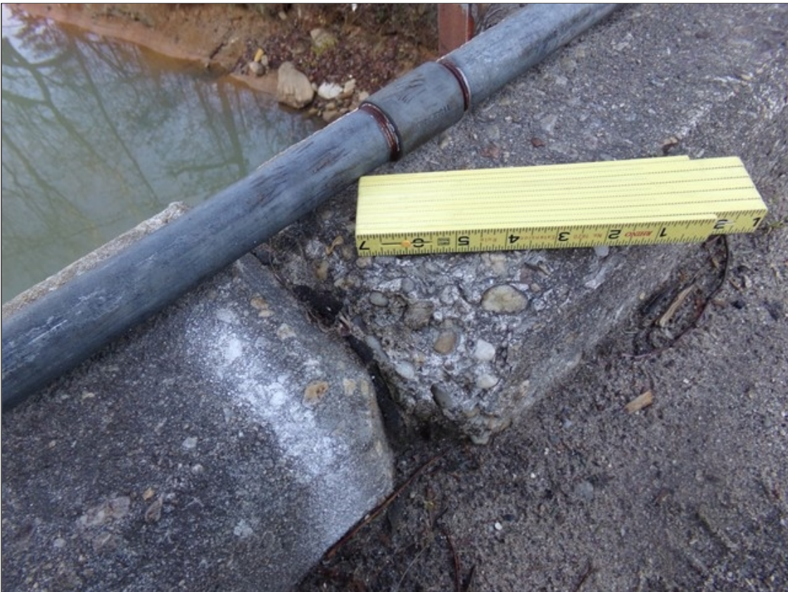
SPAN 2 LEFT RAIL - SPALL (6 INCHES X 4 INCHES X 3/4 INCH DEEP) WITH NO EXPOSED REBAR TO CONCRETE CURB AT NEAR END
