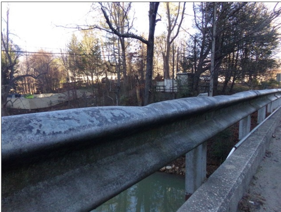
TYPICAL MINOR IMPACT DAMAGE (UP TO 15 INCHES LONG X 1.5 INCHES HIGH) THROUGHOUT TOP OF RAIL, SPAN 1 LEFT RAIL
