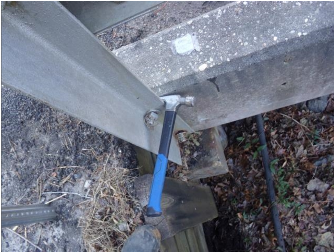
SPAN 1 RIGHT RAIL - POST 1 AND 2 LOOSE / PARTIALLY DISCONNECTED FROM CURB (PAR)
