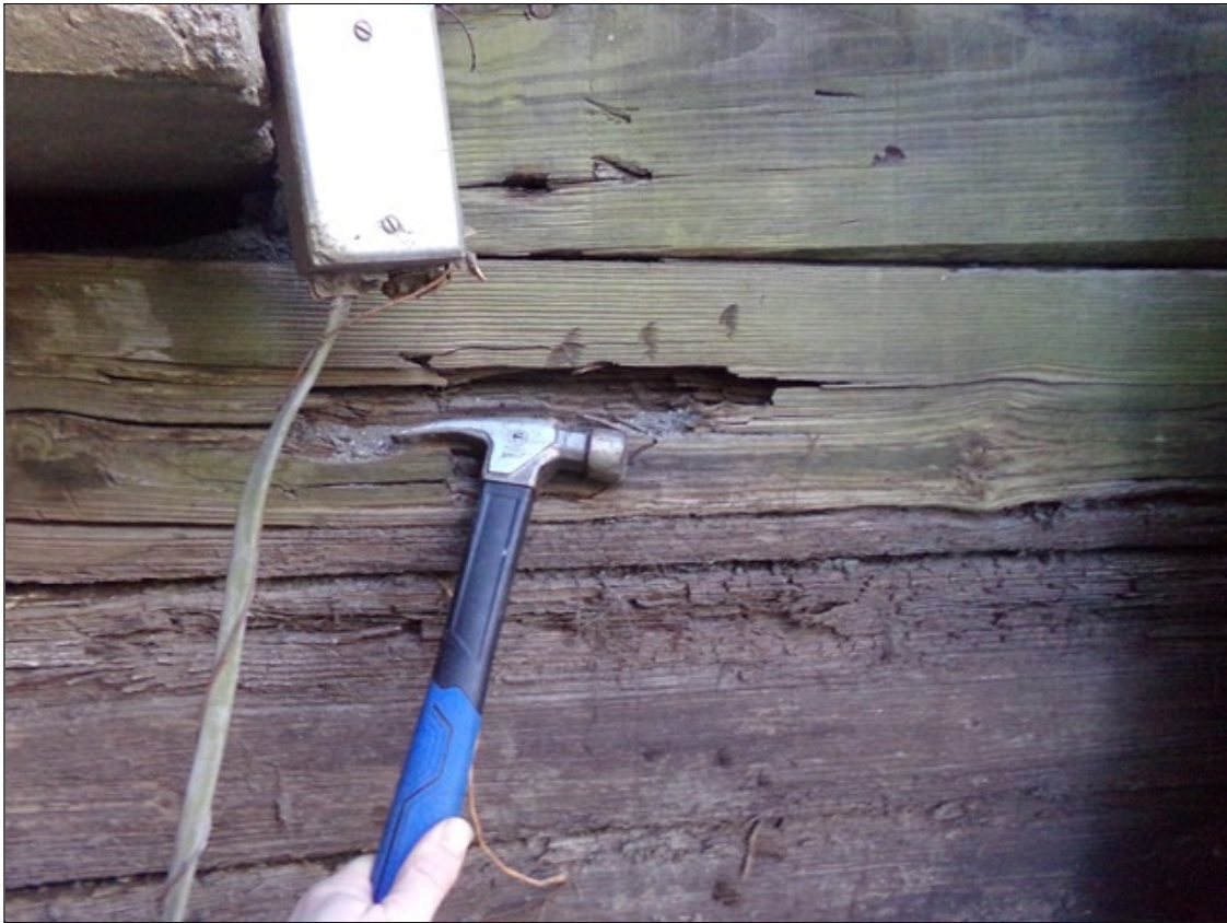
END BENT 1 ABUTMENT - INTERMITTENT MINOR DECAY (UP TO 1 INCH DEEP) AND SURFACE DECAY TO LAGGING THROUGHOUT LEFT SIDE EXTENSION (6 SQUARE FEET)
