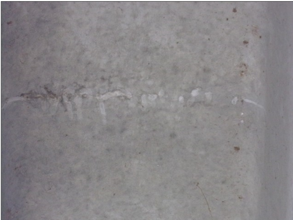
TYPICAL INTERMITTENT HAIRLINE TRANSVERSE CRACKING (UP TO FULL WIDTH) WITH MINOR EFFLORESCENCE TO BOTTOM OF SLAB BETWEEN CHANNEL LEGS, SPAN 2 BEAM 8
