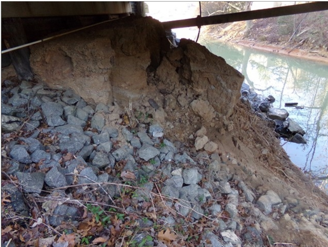
EROSION (20 FEET LONG X 10 FEET WIDE X 4 FEET HIGH) AND SOIL SEPARATION TO SLOPE BELOW SPAN 1
