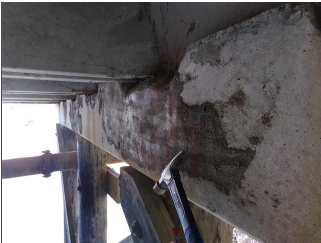
BENT 1 CAP - DELAMINATED PATCHING (3.5 SQUARE FEET) TO NEAR FACE BELOW BEAMS 5 AND 6 (PAR)
