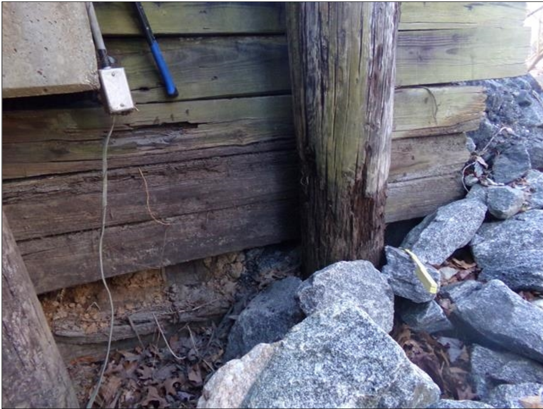
END BENT 1 ABUTMENT - LEFT SIDE EXTENSION - LAGGING UNDERMINED (10 INCHES HIGH X 6 FEET LONG) WITH SPILL-THROUGH (PAR)
