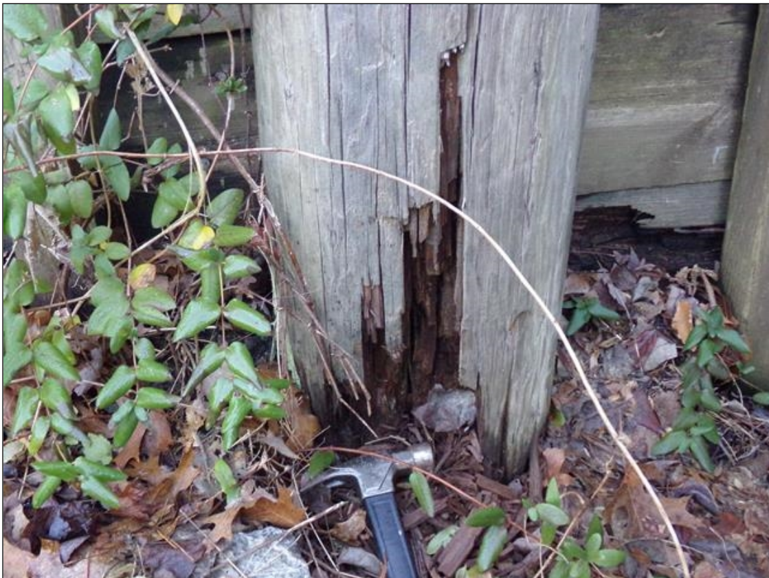
END BENT 1 ABUTMENT - RIGHT SIDE EXTENSION SOLDIER PILE - DECAY (8 INCHES WIDE X 12 INCHES HIGH X UP TO 6 INCHES DEEP) AT GROUNDLINE (PAR)
