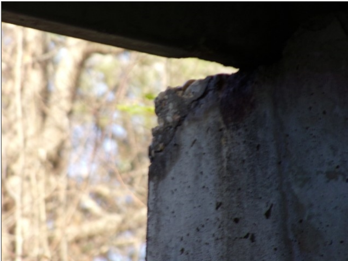
BENT 1 CAP - SPALL / DELAMINATION (8 INCH X 4 INCH X 1/2 INCH DEEP) WITH NO EXPOSED REBAR TO NEAR FACE AT TOP LEFT CORNER OF CAP
