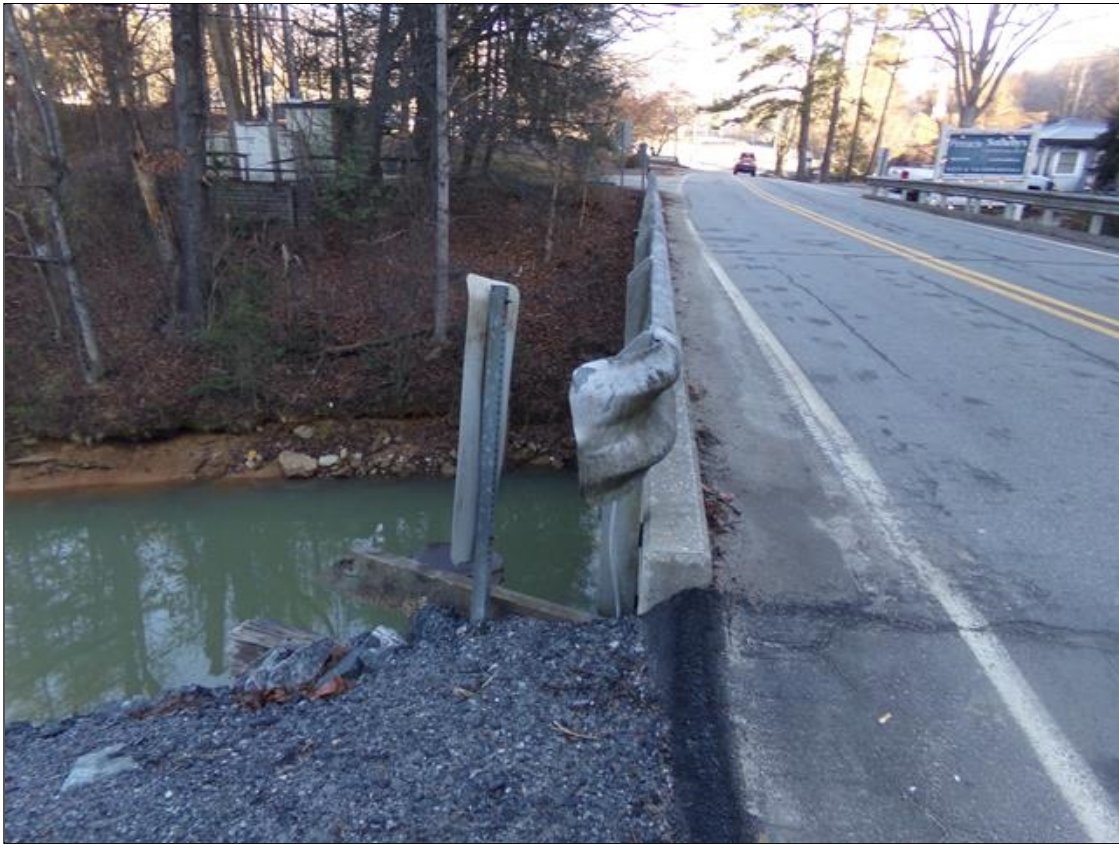
SOUTHWEST DELINEATOR - TWISTED, NOT VISIBLE FROM APPROACH (PAR)
