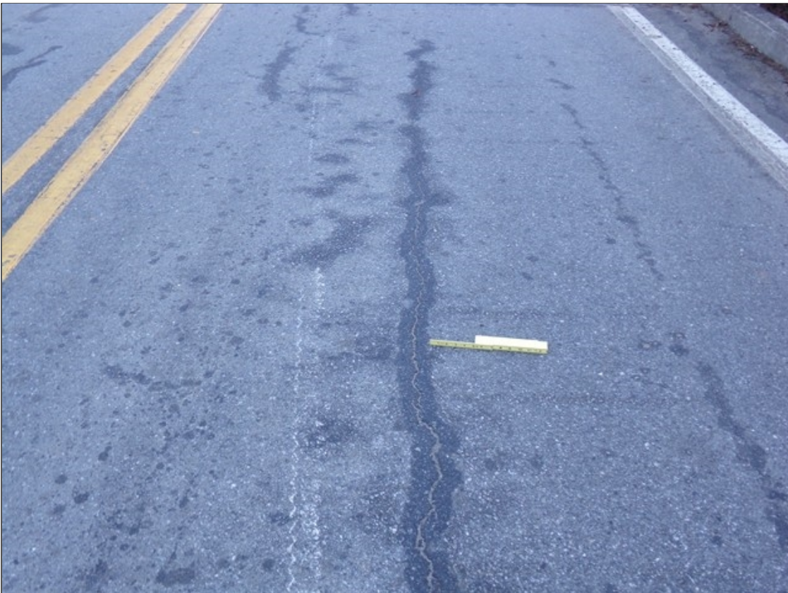
TYPICAL INTERMITTENT OPEN CRACKING (1/4 INCH X UP TO FULL LENGTH) THROUGHOUT ASPHALT WEARING SURFACE, SPAN 1 NORTHBOUND LANE
