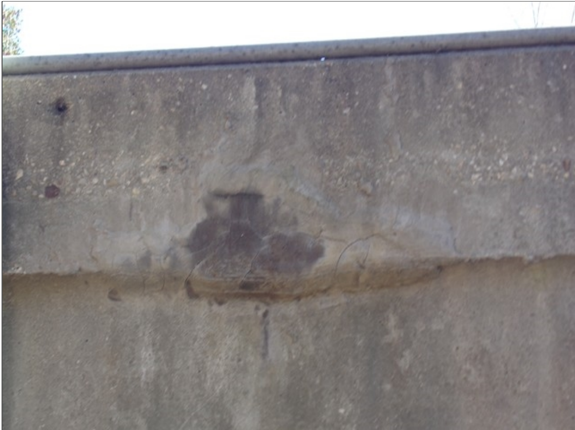
SPAN 3 BEAM 1 - DELAMINATED PATCH (24 INCHES X 12 INCHES) TO LEFT SIDE OF TOP FLANGE AT 4 FEET FROM NEAR END
