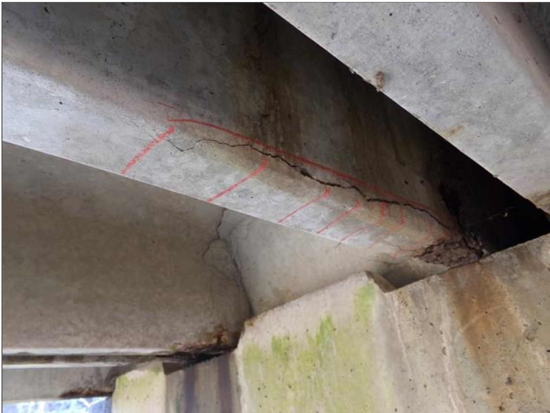
SPAN 3 BEAM 9 - DELAMINATION (20 INCHES LONG X 3 INCHES WIDE X 2 INCHES HIGH) TO LEFT LEG AT NEAR END (PAR)
