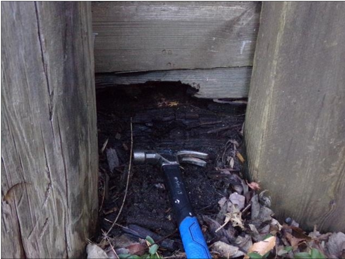
END BENT 1 ABUTMENT - DECAY (12 INCHES LONG X 8 INCHES HIGH X UP TO FULL DEPTH) TO RIGHT SIDE EXTENSION AT GROUNDLINE, ADJACENT TO SOLDIER PILE (PAR)
