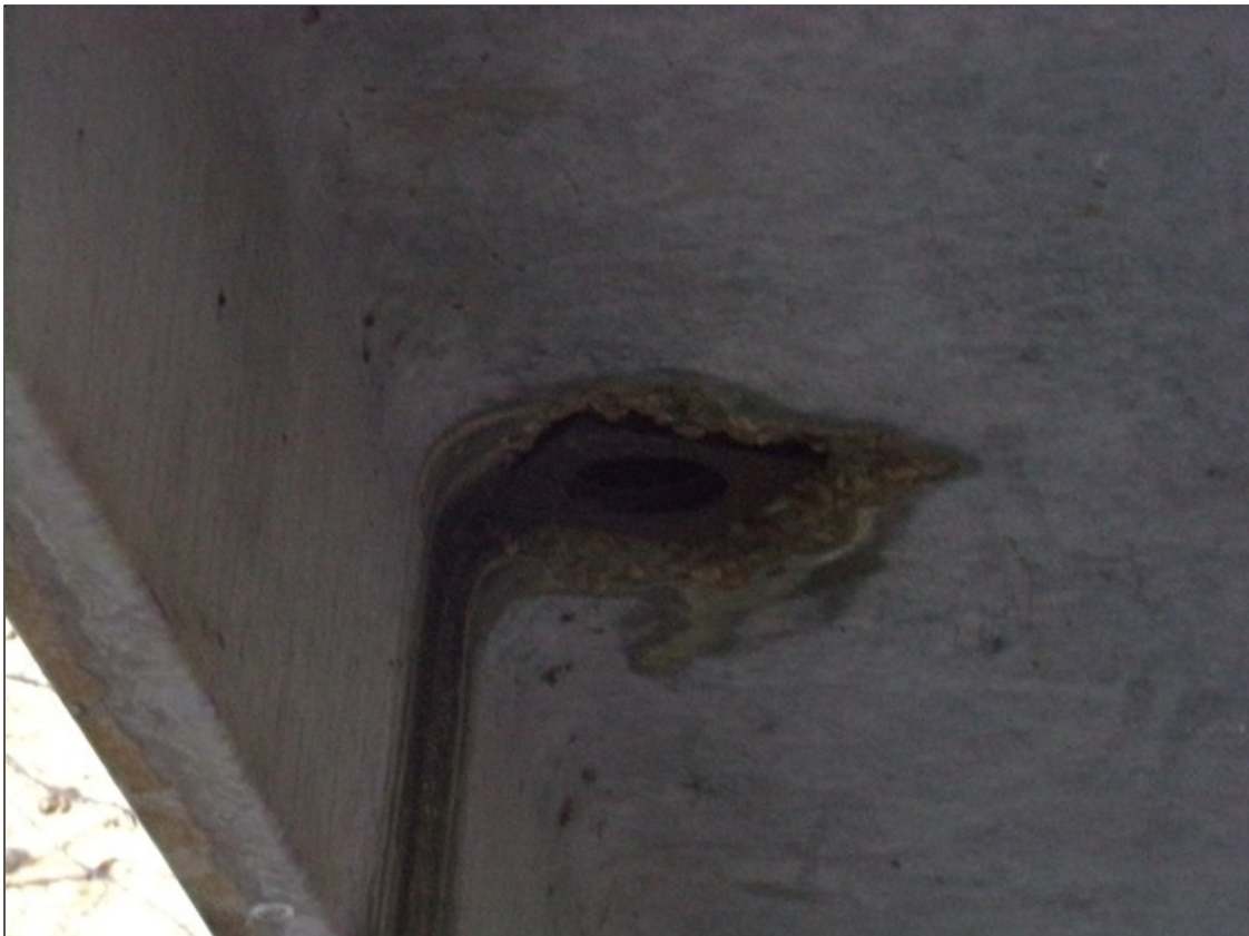
TYPICAL SPALLING (UP TO 16 INCHES X 10 INCHES X 1/2 INCH DEEP) WITH NO EXPOSED REBAR AT UNDERSIDE OF DECK DRAINS, SPAN 1 BEAM 1
