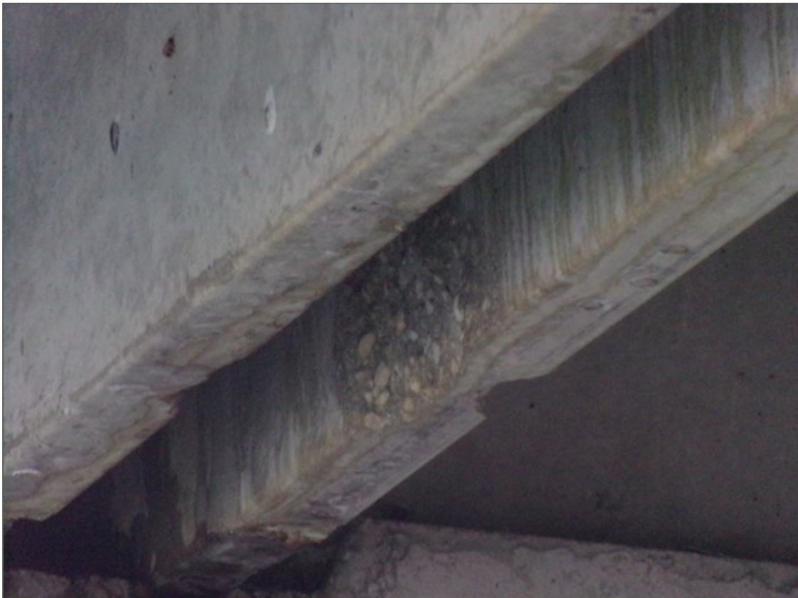
SPAN 1 BEAM 2 - SPALLING (UP TO 9 INCHES X 5 INCHES X 1/2 INCH DEEP) WITH NO EXPOSED REBAR TO BOTH FACES OF LEFT LEG AT 2 FEET FROM FAR END
