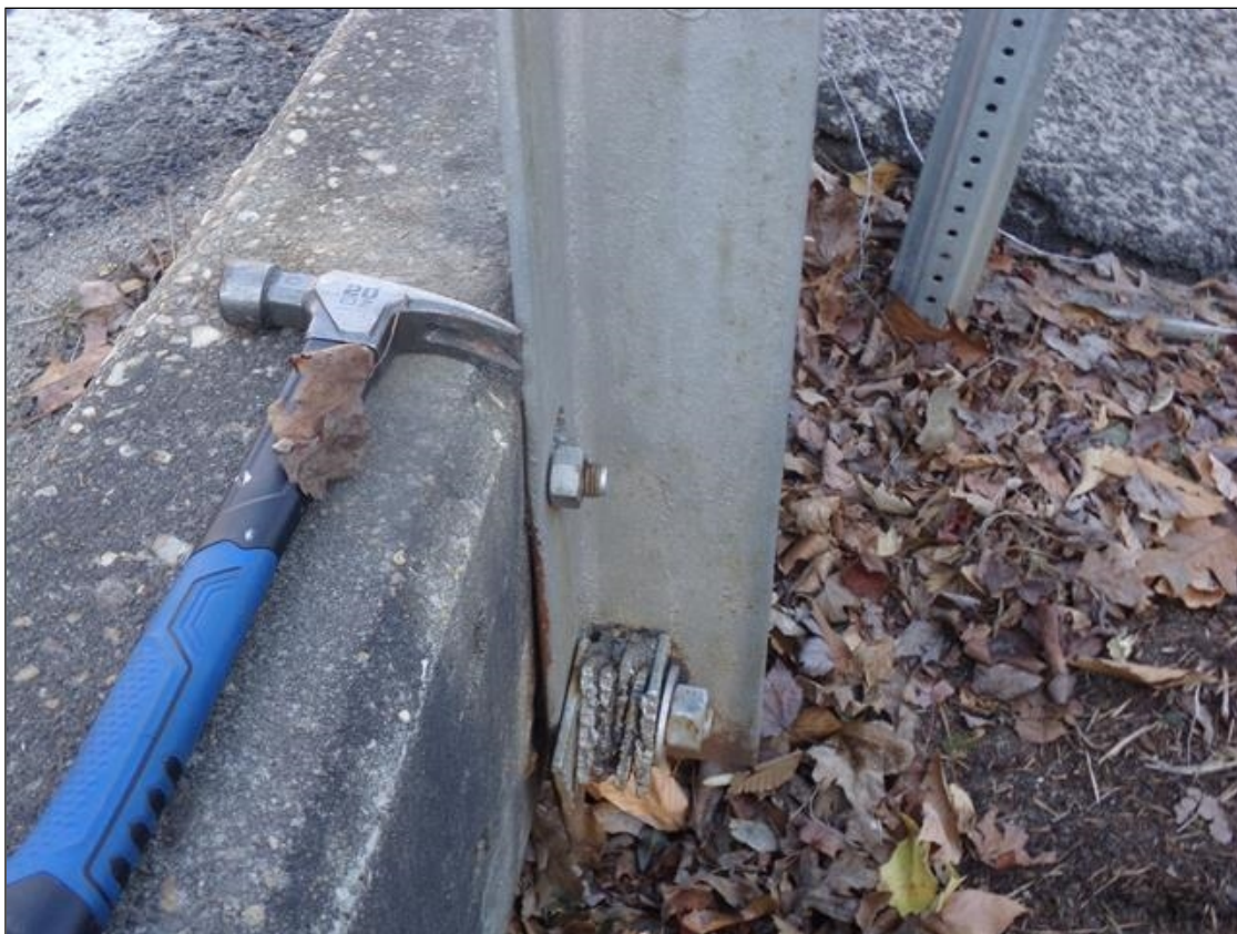
SPAN 3 RIGHT RAIL - POST 5 AND 6 LOOSE / PARTIALLY DISCONNECTED FROM CURB (PAR)
