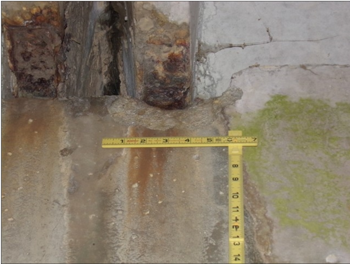
BENT 2 CAP - SPALL (6 INCHES X 3 INCHES X 1/2 INCH DEEP) WITH NO EXPOSED REBAR TO FAR FACE BELOW BEAM 8 RIGHT LEG
