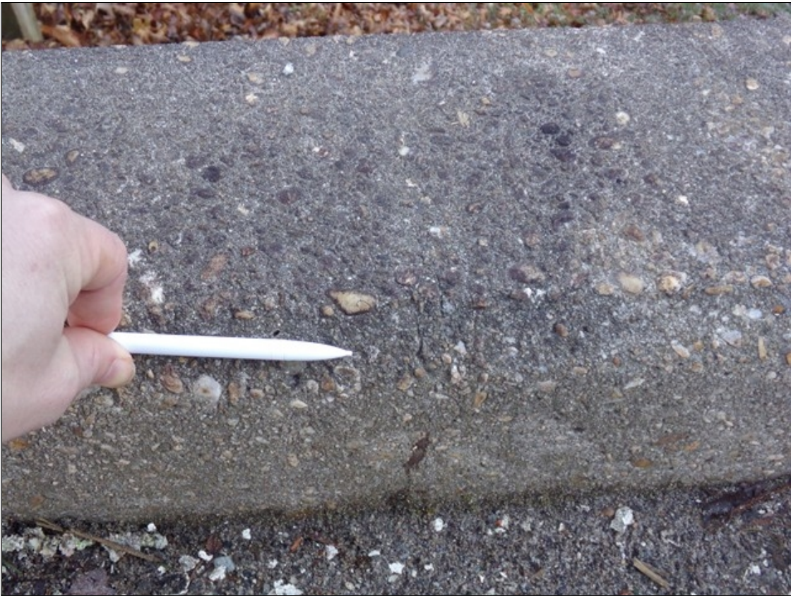
TYPICAL INTERMITTENT VERTICAL 1/32 INCH CRACKING (UP TO FULL HEIGHT) THROUGHOUT CONCRETE RAIL CURBS, SPAN 2 RIGHT RAIL
