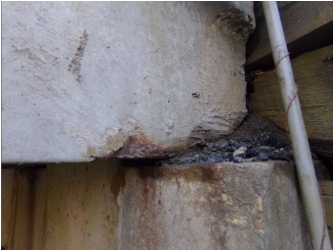
SPAN 1 BEAM 1 - SOUND PATCHING (8 INCHES X 5 INCHES) AT LEFT FACE OF LEFT LEG OVER NEAR BEARING (PREVIOUS PAR)
