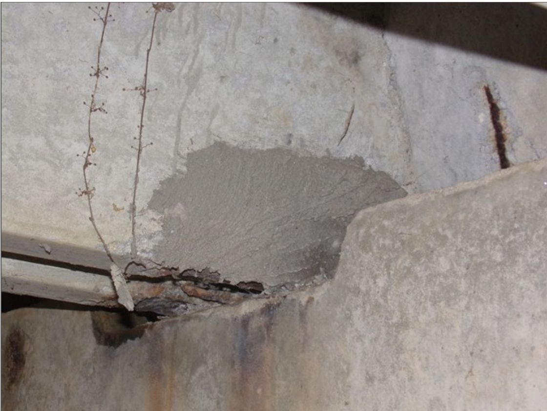
SPAN 1 BEAM 4 - SOUND PATCH (8 INCHES X 5 INCHES) TO LEFT FACE OF RIGHT LEG AT NEAR END (PREVIOUS PAR)
